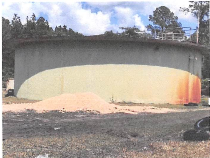
Waste Water Holding Tank
