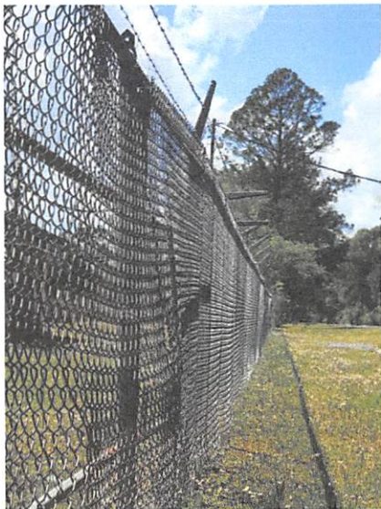
Fencing around perimeter of land needs replacing
