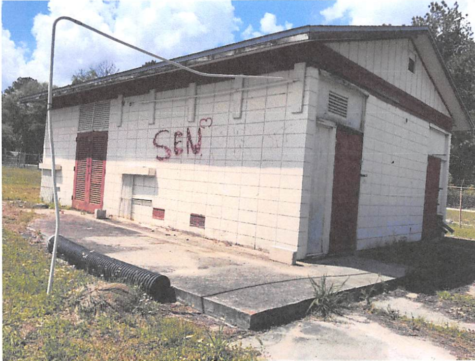
Primary lift station
