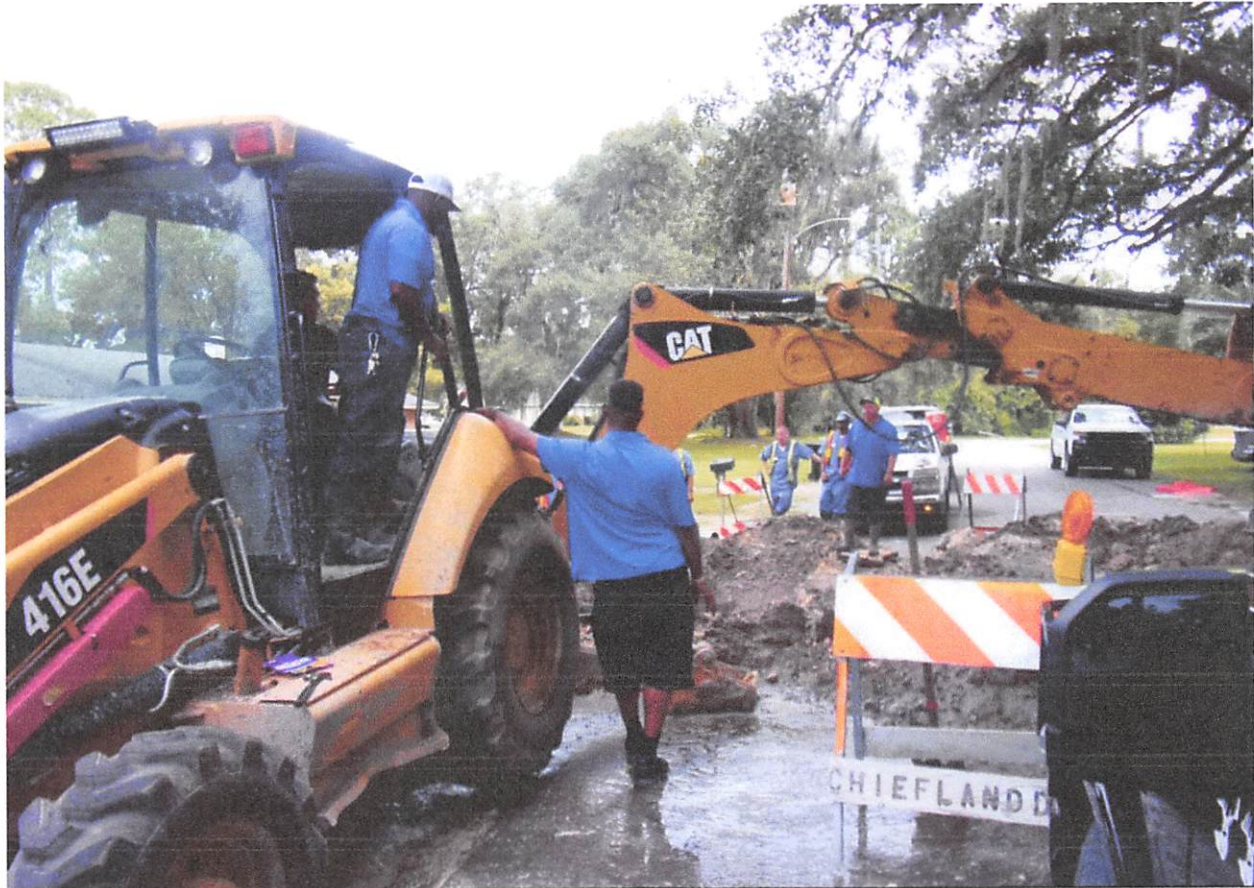
Water line leak and struggle with finding the turn off valve in an old system that is not mapped.
