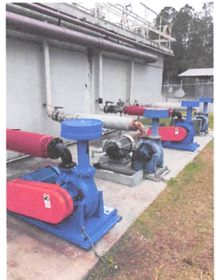
Wastewater Treatment Plant new motors
