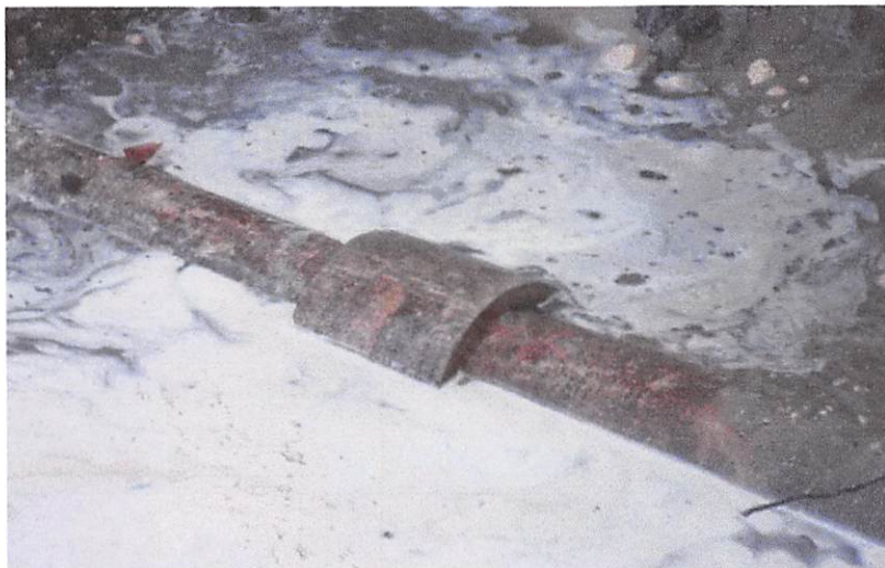
Old asbestos laden line with crack and no turn off valve to shut water off
